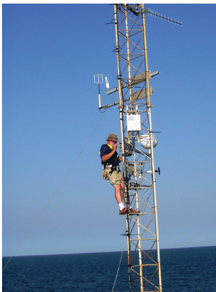
ARL scientist deploying an ET Probe on a tower at the end of a 560 meter long pier in Duck, NC during August 2009. (image: NOAA)
